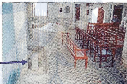
The structural engineers have dug a 10-foot hole along the north wall (see arrow) to determine the strength of the foundation of the walls and columns. From that excavation they have discovered a street which existed underneath where the synagogue was built.
